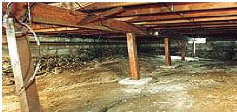
Crawlspaces with Exposed Soils or that Lack Vapor Barriers will typically have moisture / growth issues
